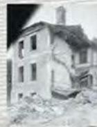
Tabbs House Photograph By the time American photographers first visited Dumfries in the 1830s, it was beyond repair. A few weeks after the photograph was taken, the house was demolished.
